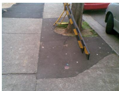
Concrete - poor condition
